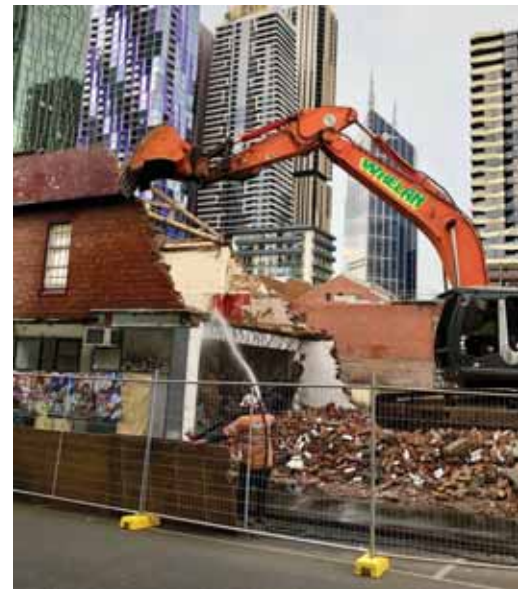
Demolition of early twentieth inter-war commercial buildings, south side of Therry Street between Queen and Elizabeth Streets (nos 97-141), 18 January 2019 (photo C. Sowerwine).
